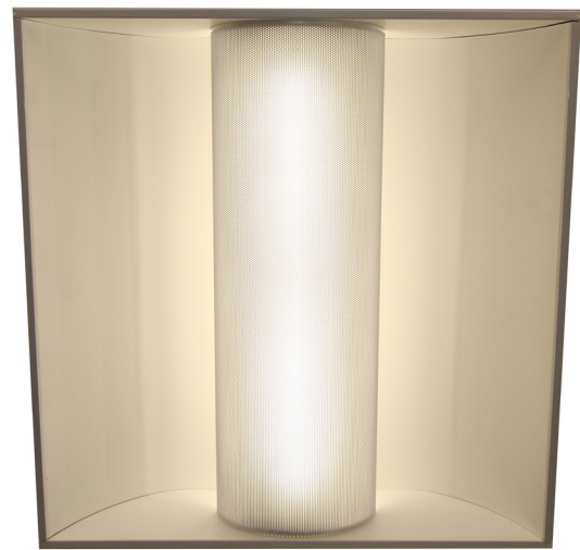
Retrofitted Center Basket Fixture
